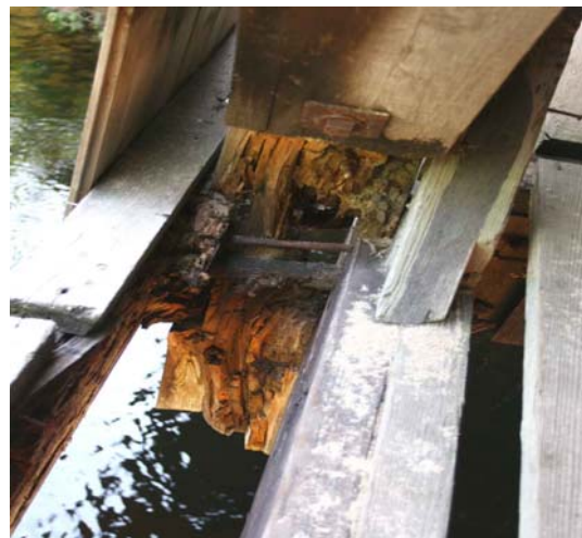
Close-up view of decayed horizontal chord and base of a vertical kingpost.
