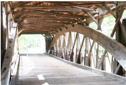
Interior View of Whittier Bridge shows pronounced tilt of supporting arches leftward, toward downstream side.
