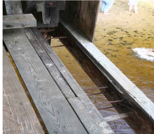
Decay has destroyed 20 feet of main center beam of lower supporting chord on the downstream side, exposing rusted steel tie-rods and a hardwood trunnel between the chord's remaining side-planks. Supporting arch now carries full load, resulting in tilt and deformation of curvature.
